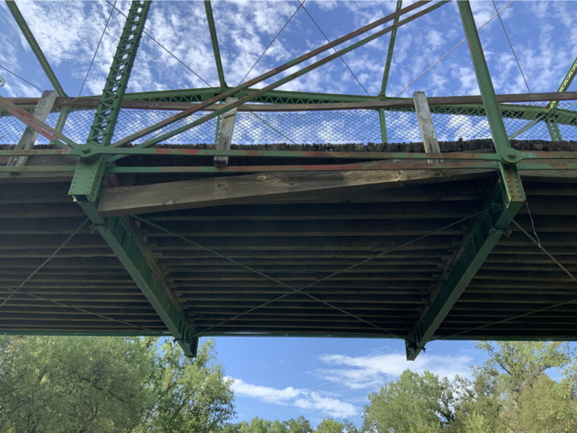
Photo #5 Stringer 17 has completely migrated off of Floor Beam 5
