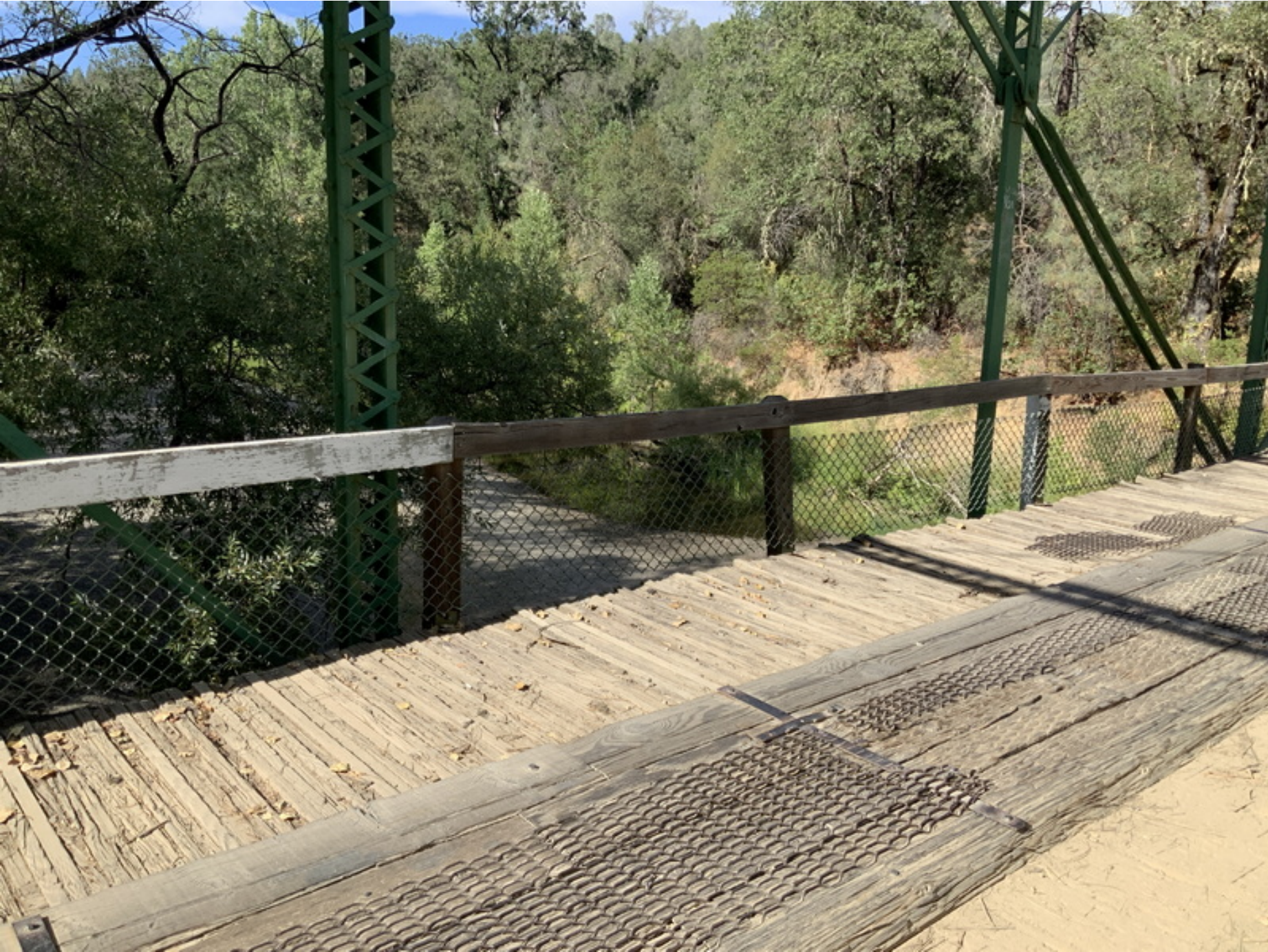
Photo #4 Replaced missing section in the left timber rail. Far right side of photo replaced
